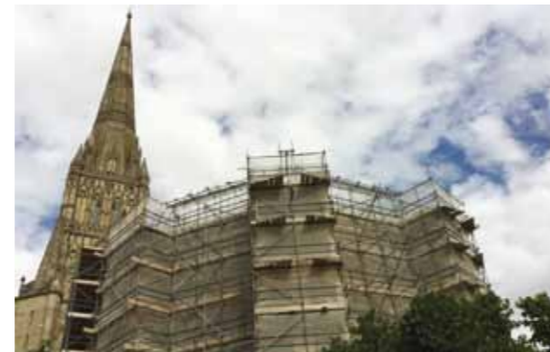
Major Repair Programme work begins on the Chapter House thanks to a generous anonymous donation.
